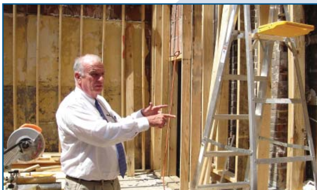
St. Thomas Community Health Center President and CEO Don Erwin describes the renovations made to the facility.
